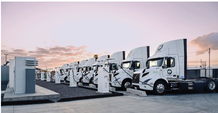
Completed in April 2024, the Denker Hub is the largest heavy-duty truck charging hub in North America, powered by a self-sufficient microgrid with 18 MWH energy storage, 9 MW charging capacity, and 96 charging stalls.
